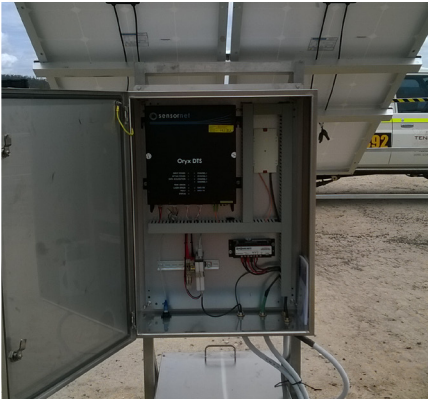
Oryx+ DTS unit installed onsite
