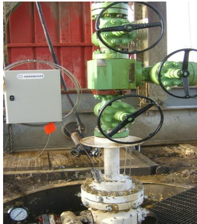
Figure 4 Surface Junction box for fiber optic terminations
